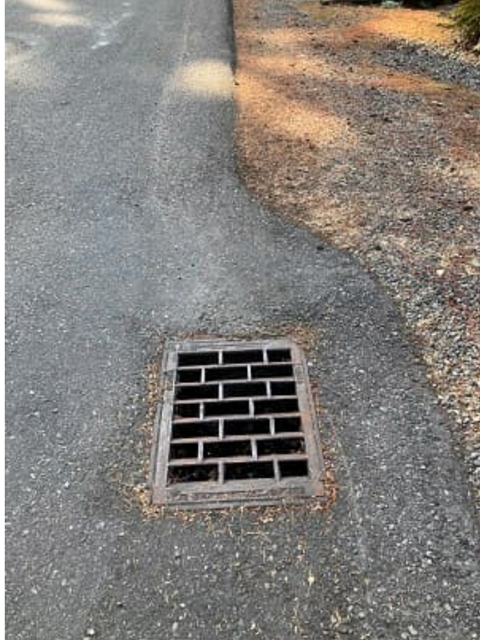
Picture 1: ROW in front of 3443 72 nd Place SE Storm will extend south from project site to this catch basin.
