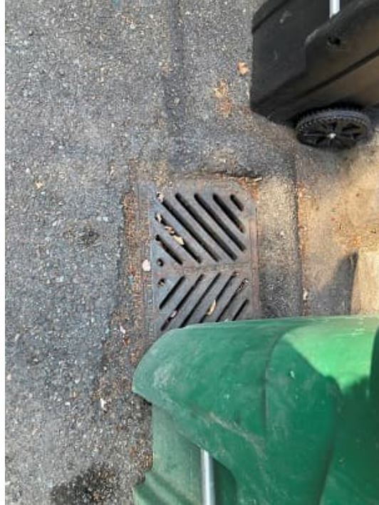
Picture 18 ROW in front of 3698 72 nd Place SE From this catch basin water heads toward the west.
