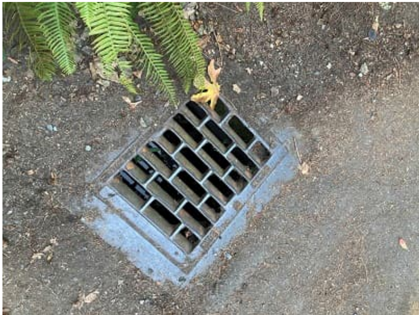
Picture 13 ROW at the NE corner of 73 rd Avenue SE and SE 38 th Street At this CB the storm drain makes a turn east under the SE 38 th Street ROW
